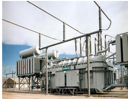
Phase shifting transformer for power flow control
