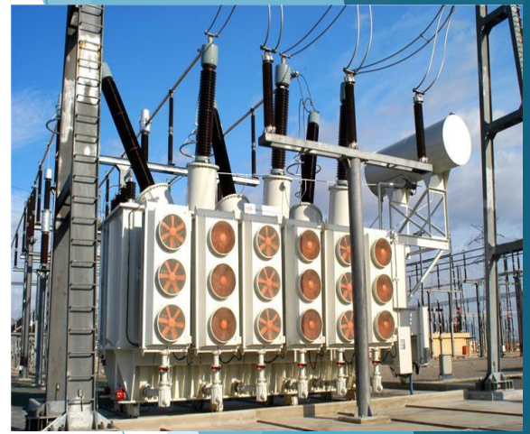
Substation power transformer
