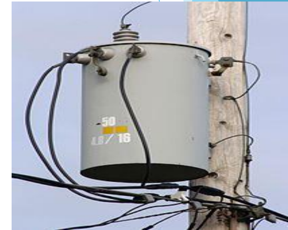
Pole mounted single phase distribution transformer
